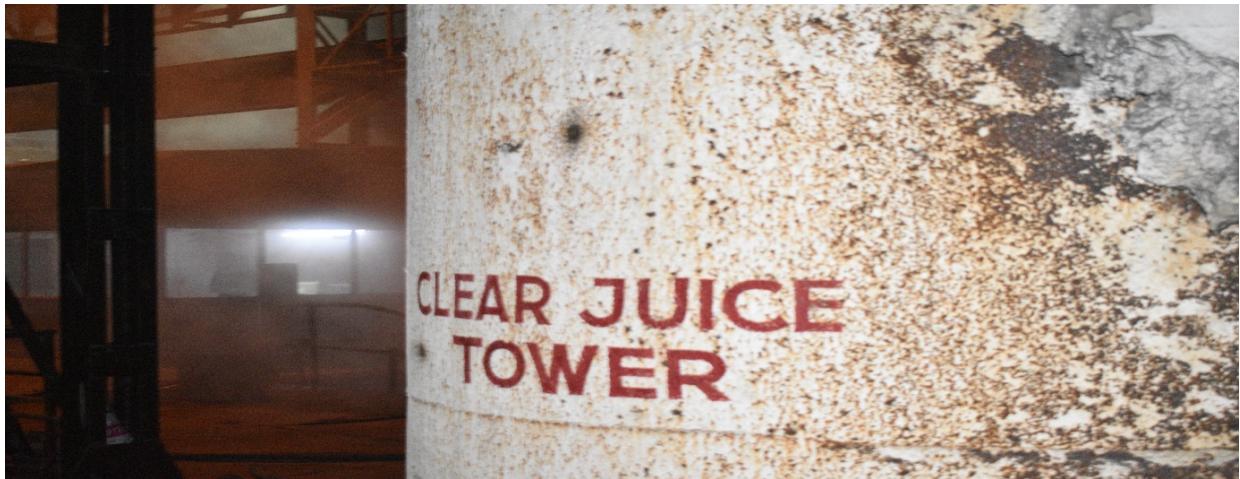
Image: Clear juice collection tower at Uttam Sugar Mills Ltd.
