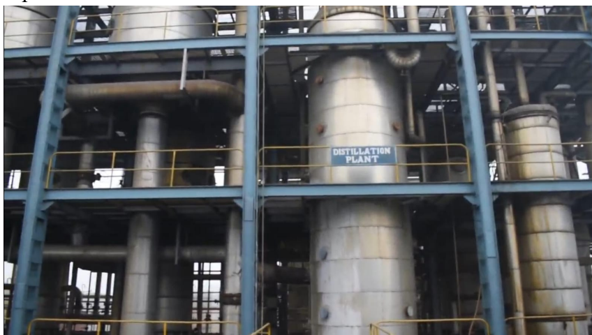
Image: Distillation process plant at Nanglamal Sugar Complex, Mawana Sugars.
